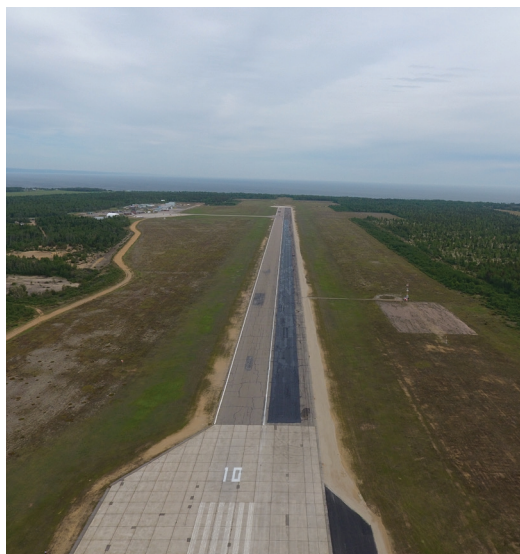
Aerial photo of Runway 10 at the Baie-Comeau Airport during the rehabilitation work on the south side of the runway in June 2018
