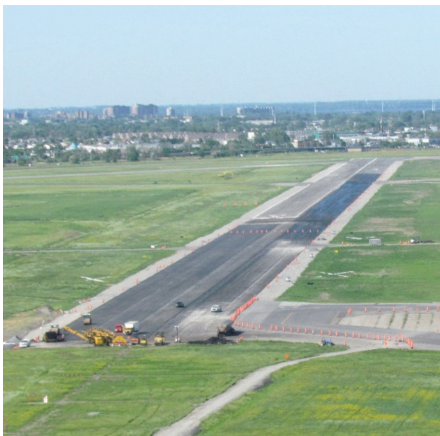
Aerial photo of the runway markings used for Runway 24R at the Montréal/St-Hubert Airport during the 1st phase of construction
