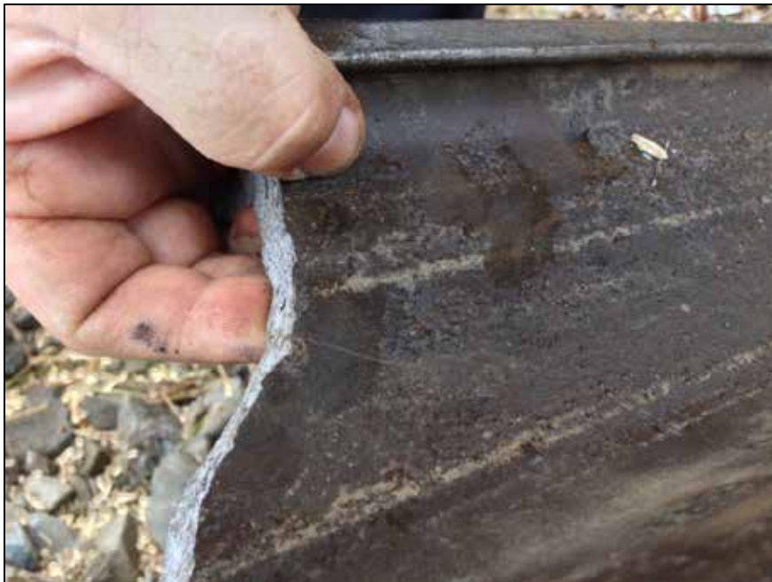
Photo 1. Wheel flange marks on the web of the high rail
