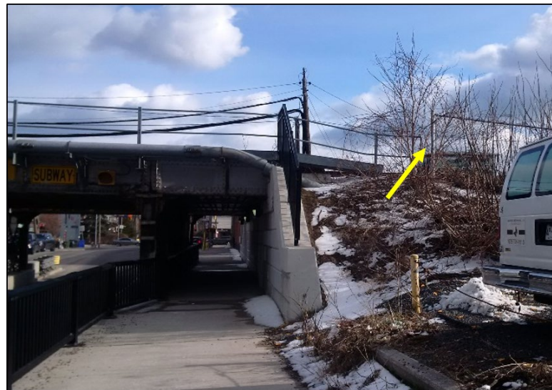
Figure 4. Gap in the fencing at the Howland Avenue grade-separated crossing, where the teenagers accessed the right-of-way (Source: TSB)
