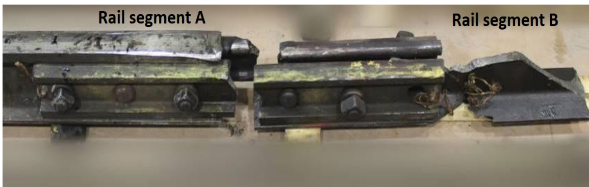
Figure 12. South rail joint 1, field-side view with 132/136 RE standard joint bar. Note yellow paint marking defective joint for repair (Source: TSB)
