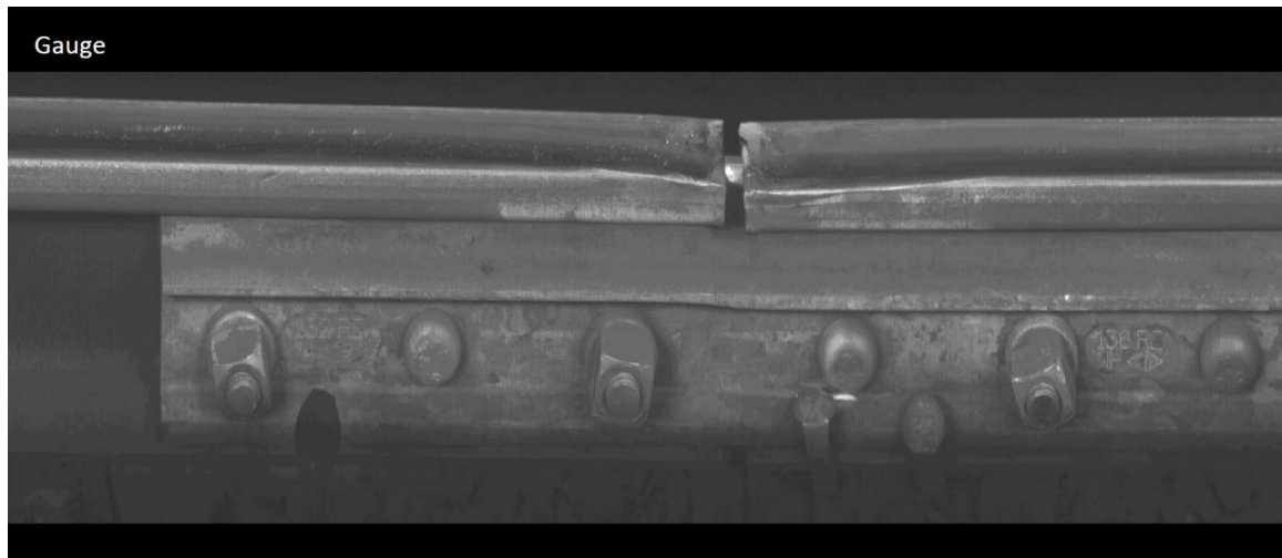
Figure 8. Gauge-side compromise joint bar (Mile 197.4751) showing rail head end batter (Source: Canadian National Railway Company)
