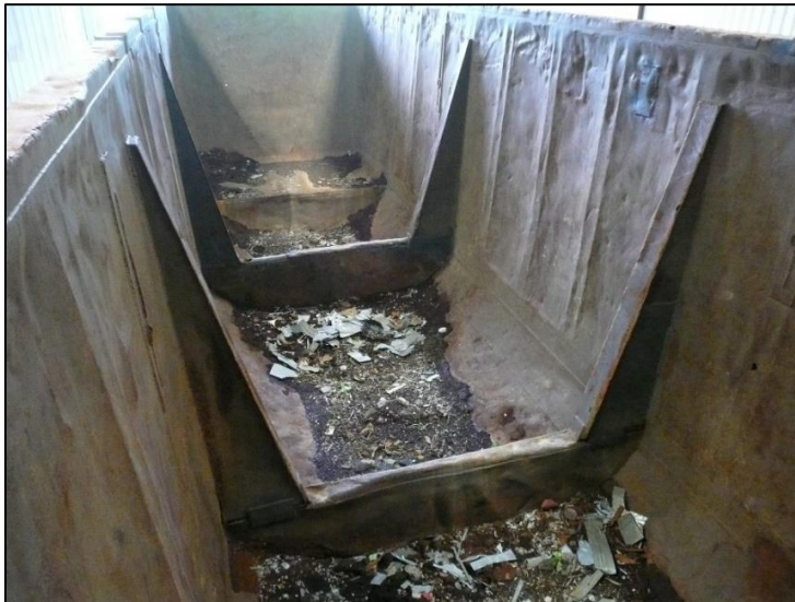
Figure 24. Car DJJX 30156, as modified, with 2 large steel u-channels fabricated inside the car to compensate for the removal of the 2 upper reinforcement crossbars (Source TSB)
