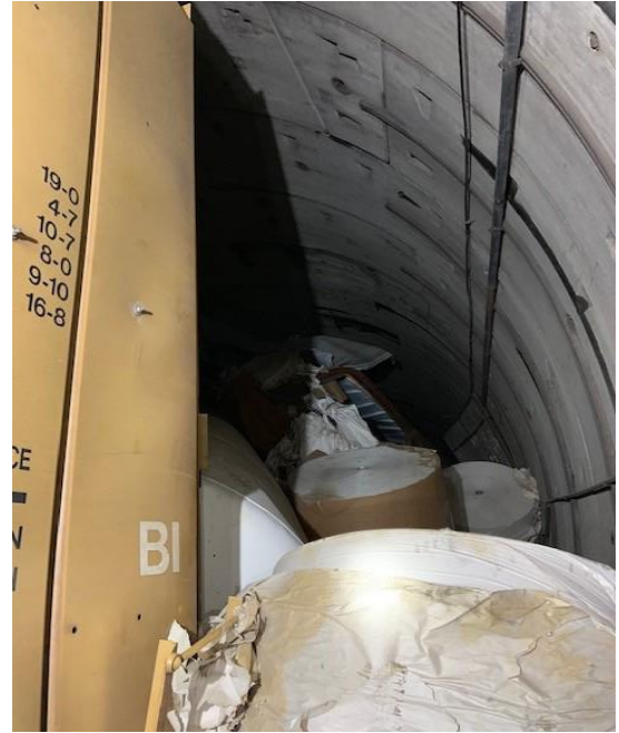
Figure 11. Second example of blocked tunnel on the U.S. side (Source: Environmental Protection Agency)
