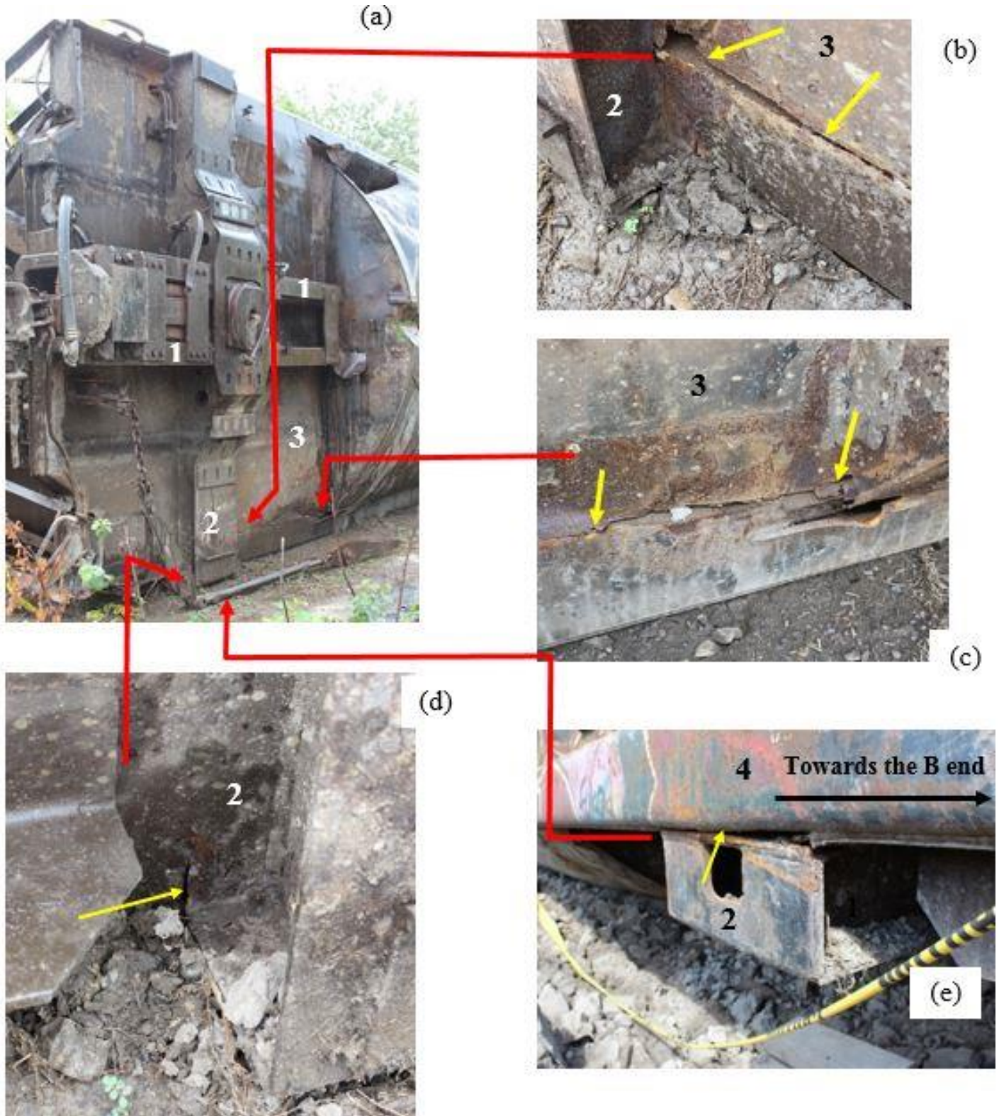
Figure 28. Car DJJX 30478 B-end underframe . Photo (a) shows the bottom of B-end, including the stub sill and car body bolster; photos (b) and (c) are close-up views of cracks found on the shear plate (yellow arrows) in photo (a); photos (d) and (e) show cracks found in the joint between the car body bolster and side sill in photo (a) (Source: TSB)
