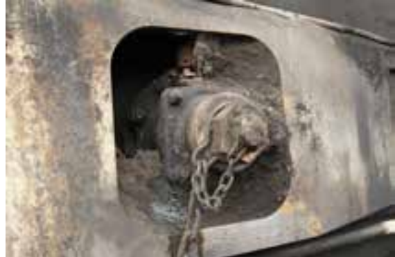
(h) Close-up showing seepage from BOV
