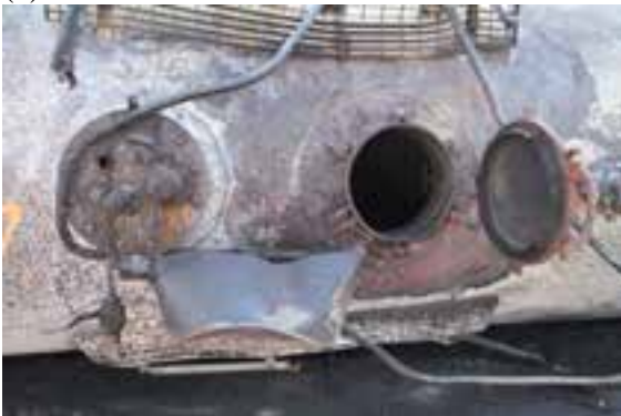
(g) Top fittings and manway
