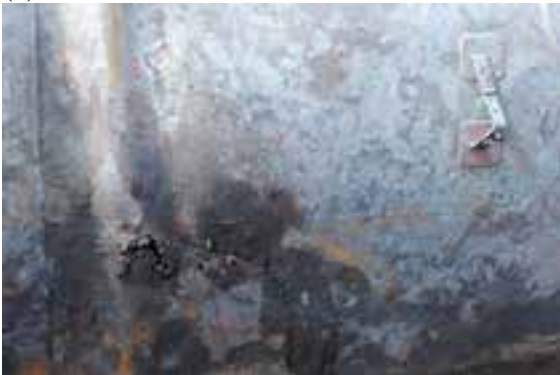
(e) Burn-through on left side of shell – see arrow in (d)
