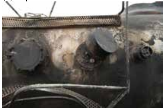
(f) Manway, top fittings and PRD
