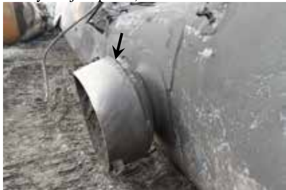
(f) Detail showing damaged housing wall (arrow)
