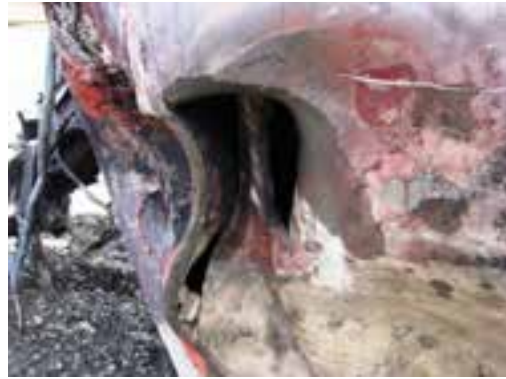
b) Close-up showing the ruptures indicated by the arrow in (a)
