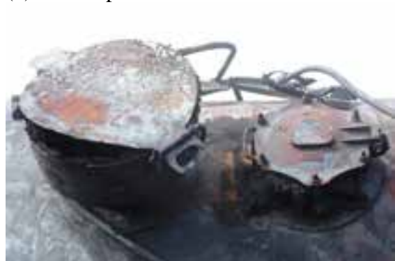
(f) Top fittings and manway
