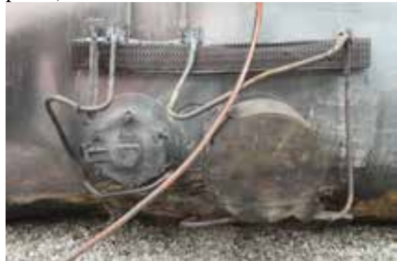
(f) Top fittings and manway
