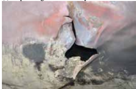
(h) Close-up of puncture in shell (RSI-AAR Safety Project photo)
