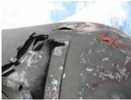
(b) Close-up showing small ruptures at B end
