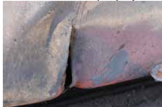
(f) Close-up of rupture arrowed in (e)
