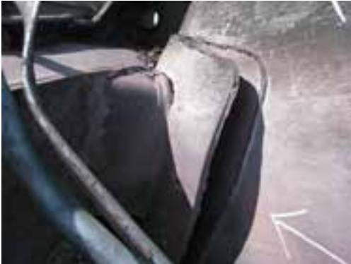
(c) Close-up showing front sill pad separation - see lower arrow in (b)
