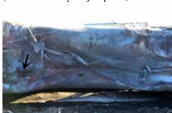
(f) Burn-throughs and puncture (arrow) on shell (RSI-AAR Safety Project photo)
