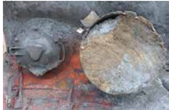
(f) Manway and top fittings
