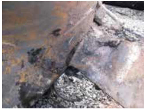
(b) Close-up showing separation at B end head brace to front sill pad fillet weld - see arrow in (a)
