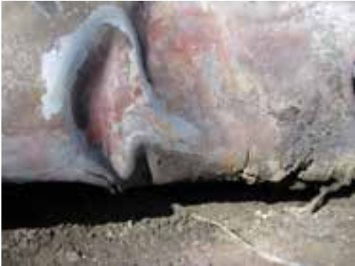
(c) Shell damage in the area indicated by the arrow on (b)
