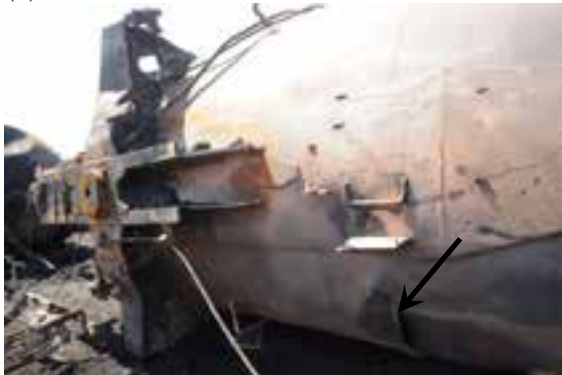
(e) Rupture in shell (arrow)
