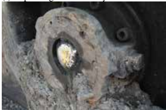
(h) Close up showing light seepage from BOV
