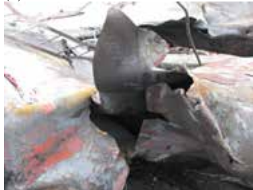
(f) Shell rupture adjacent to manway
