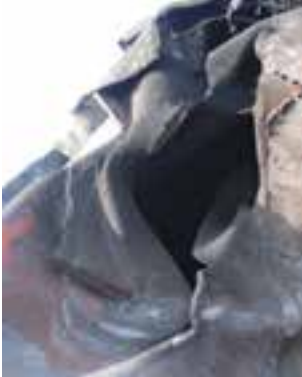
(c) Close-up showing rupture at shell-to-head weld at B end
