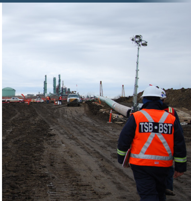
PHOTO 15. TSB investigator on site of the Sherwood Park pipeline occurrence
