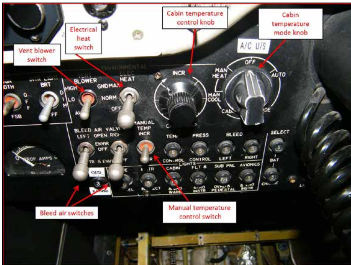
Photo 2. Environmental control panel
