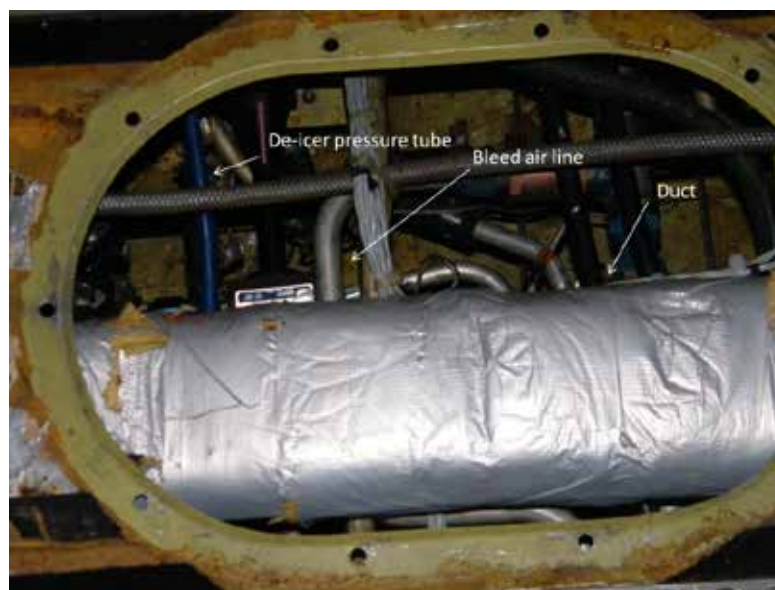
Photo 3. Hot air duct, de-icer pressure tube and bleed air line under the right side of the floor during tests
