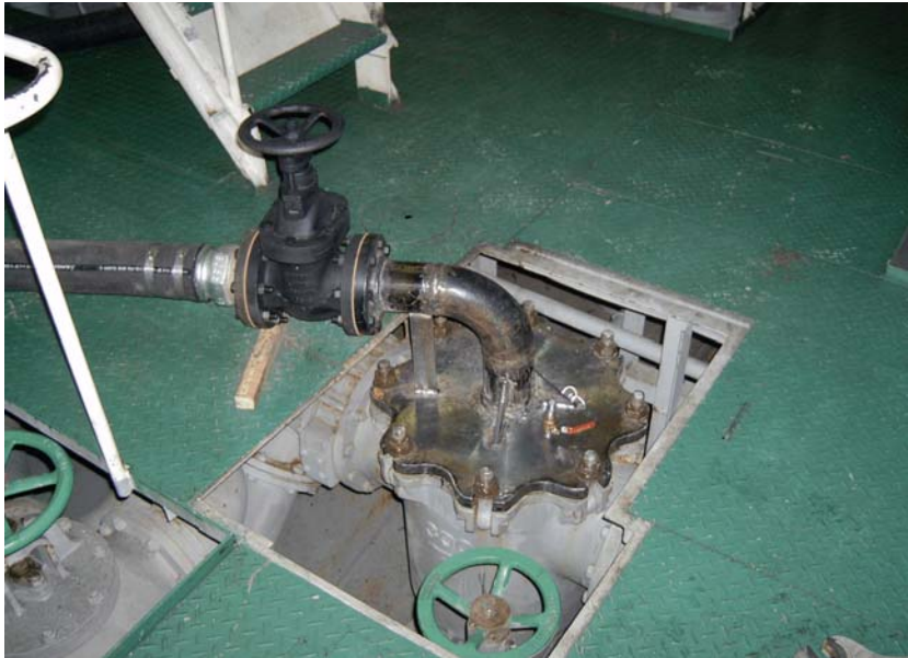
Photo 4. Temporary pipe connected to sea strainer returning main engine cooling water directly to sea chest.
