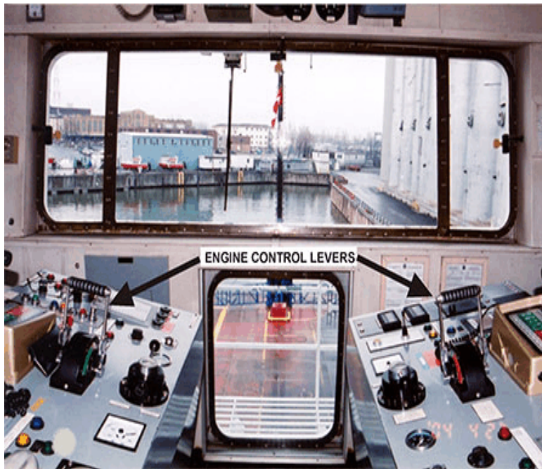
Photo 2. Bridge control consoles, looking either forward or aft
