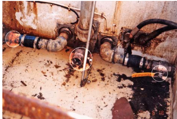
Photo 5. View in the lazarette showing sluice valves for the live-well tanks and the lazarette
