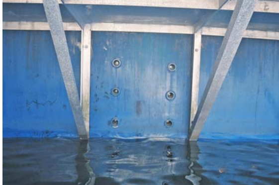
Photo 2. Exterior view of the transom under the platform showing six seawater discharge ports connected to the live-well tanks
