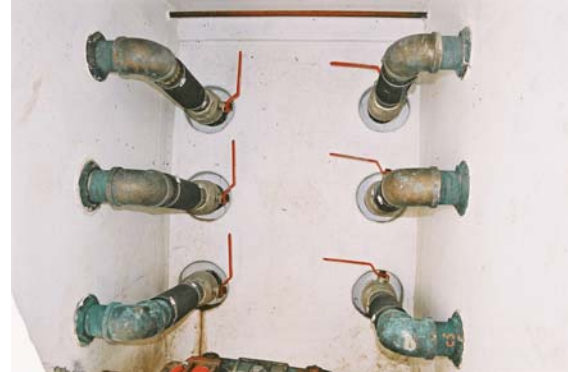
Photo 3. Interior view in the lazarette showing discharge pipes connecting the live-well tanks to the transom. Each pipe has a 76 mm valve.
