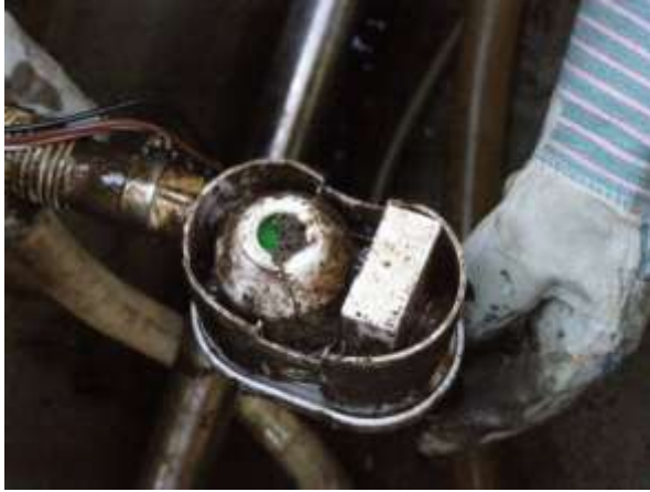
Photo 6. The electrical pump coated in oil and the impeller partly obstructed with fibre; the mounting base/ strainer is not in place
