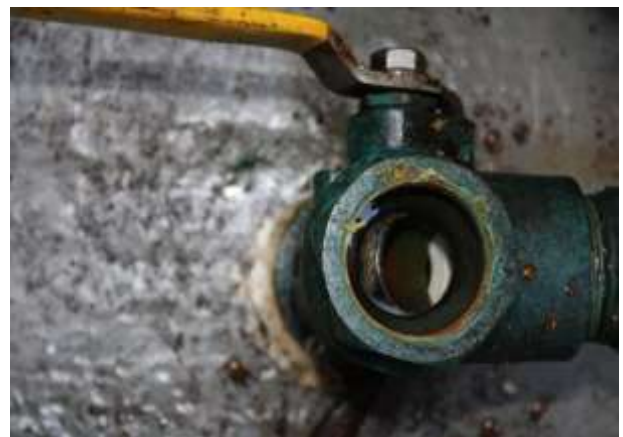
Photo 4. Three-way valve partially open to the sea
