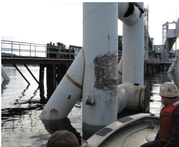
Photo 4. Port-side fender showing point of contact and missing pad
