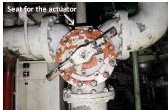
Photo 3. Sea water 3-way valve without actuator installed (this photo has been rotated 180° for comparison with Photo 2)
