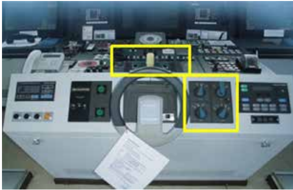
Photo 7. Nilufer Sultan bridge main console (steering control panels indicated by yellow boxes)
