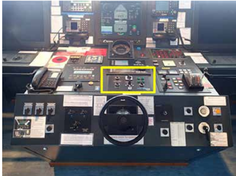
Photo 6. Manas bridge centre console (steering control panel indicated by yellow box)
