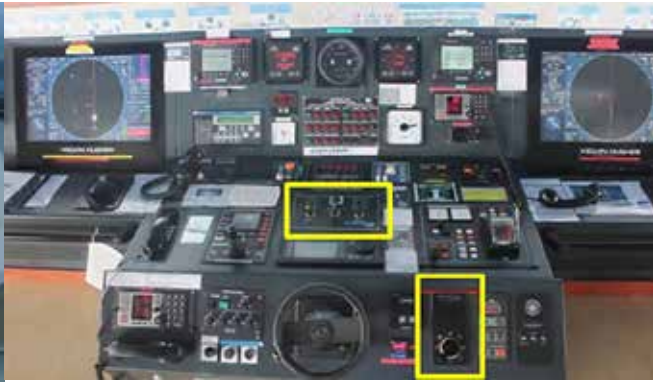
Photo 8. Mehmet A bridge main console (steering control panels indicated by yellow boxes)
