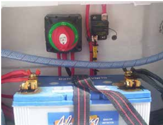
Figure 2. Builder-approved and standard battery bank arrangement in both battery compartments (Source: LeisureCAT Australia, LeisureCat 8000 Sportsfisher Owners Manual)
