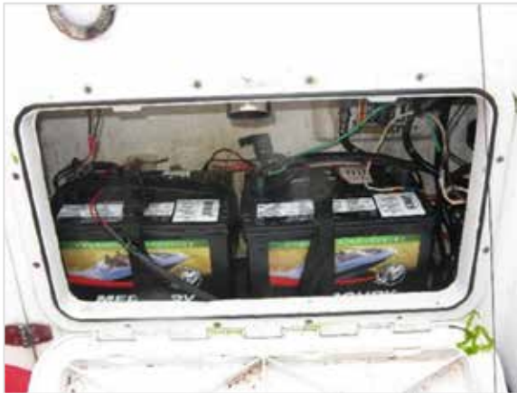
Figure 3. Modified, non-standard arrangement of battery banks in the port battery compartment
