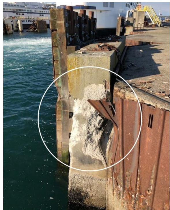
Figure 3. Damage to the concrete abutment (circled) (Source: BC Ferries, with TSB annotations)
