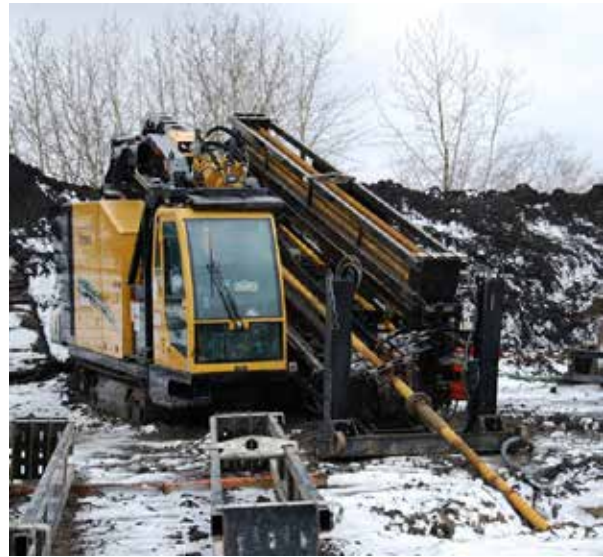
Figure 6. Drilling rig involved in the pull-through operation of the NPS 20 GRP pipeline
