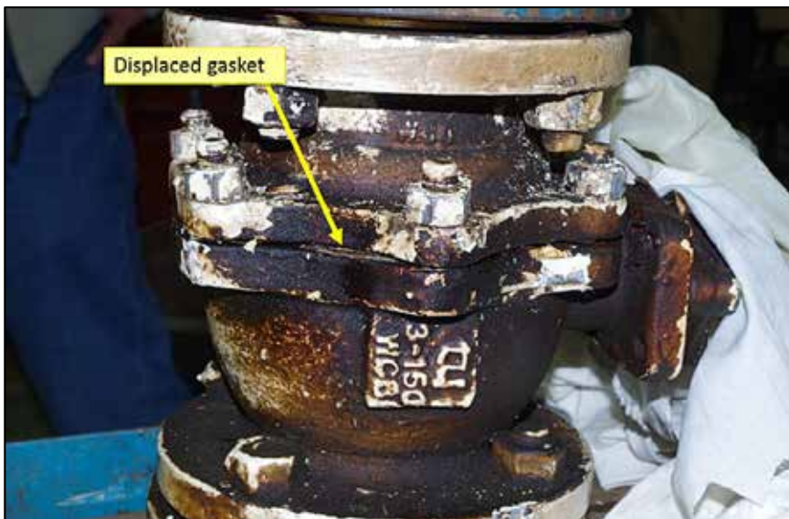
Figure 9. Displaced gasket (Source: Acuren Group Inc., with TSB annotations)
