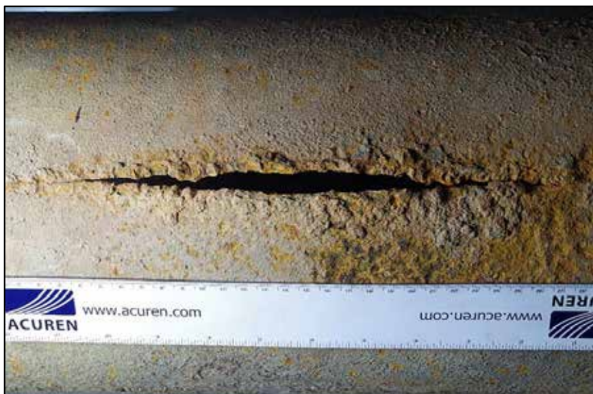
Figure 12. Split at the longitudinal seam weld (Source: Acuren Group Inc.)
