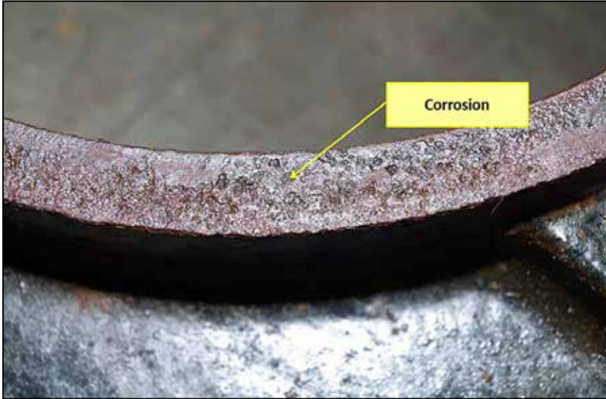
Figure 10. Corrosion at valve seat (Source: Acuren Group Inc., with TSB annotations)
