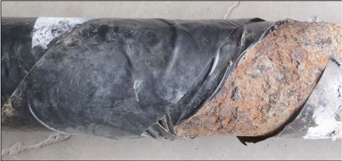
Figure 9. External pipe surface condition after the occurrence (Source: Acuren Group Inc.)
