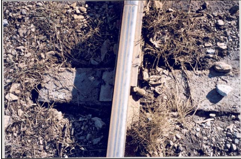
Photo 3. Fouled ballast on track G-5 in the vicinity of the derailment site
