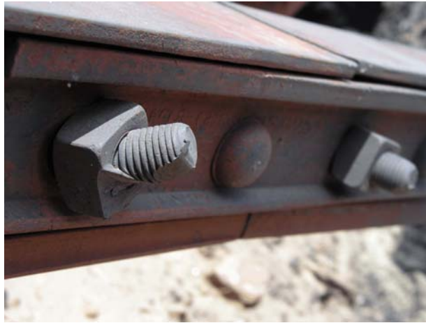
Photo 3. Impact mark on the guard rail splice bar bolt
