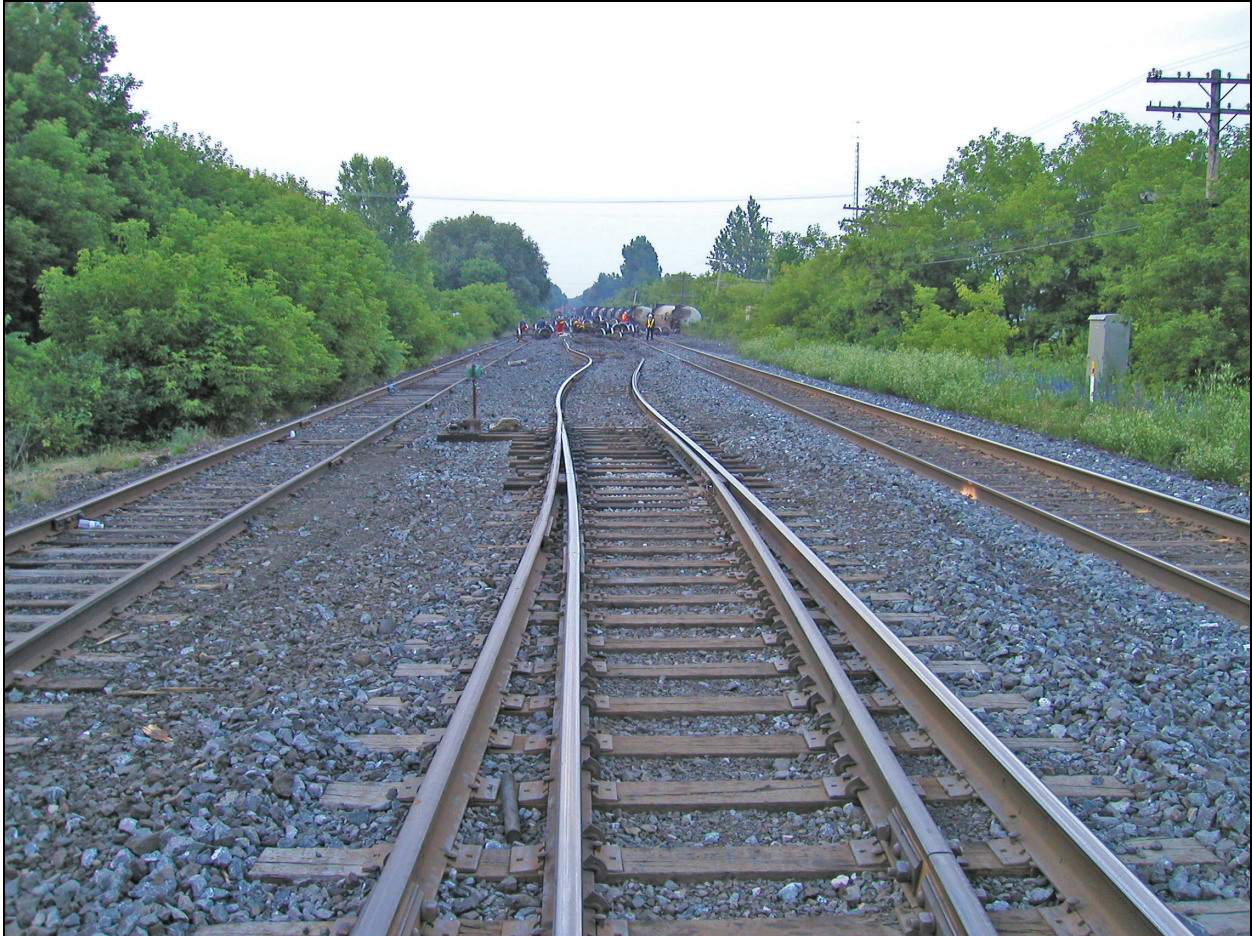
Photo 1. Derailment zone showing the track buckle
