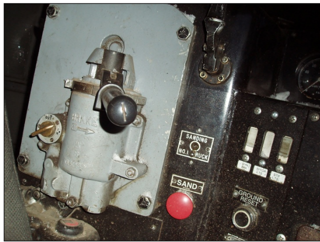
Photo 4. Automatic brake valve and brake valve cut-off cock on lead locomotive. The automatic brake valve handle is in the “handle off” position, the cut out cock is between the “in” and “out” position.
