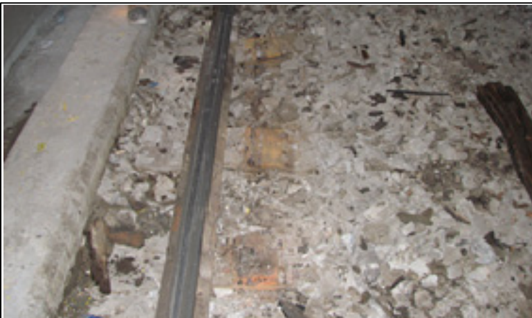
Photo 3. Lateral displacement of south rail
