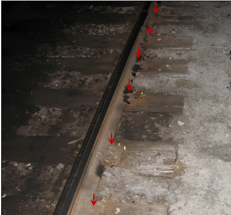
Photo 6. Locations of 10-inch tie plates with round spikes, indicated by red arrows – north rail
