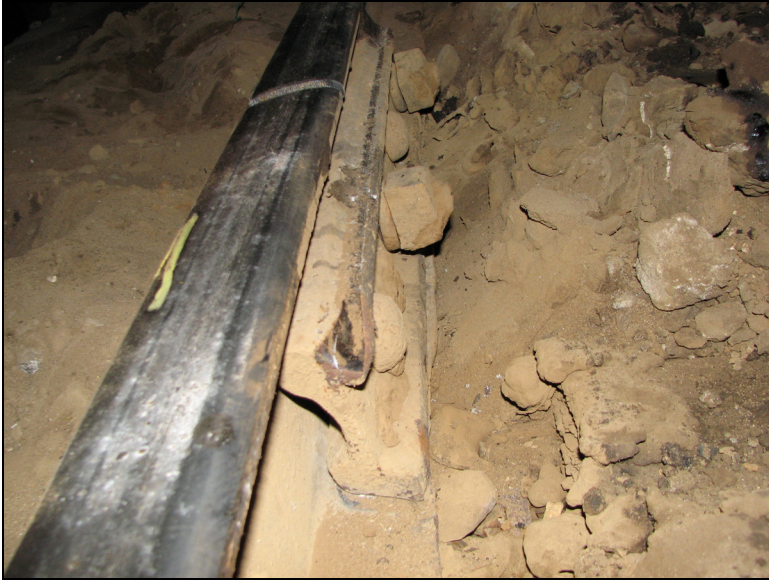
Photo 2. Marks on rail joint in south rail
