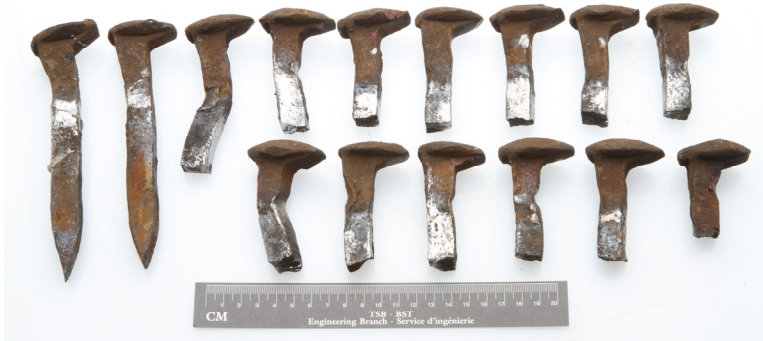
Photo 14. Track 21 broken track spikes
