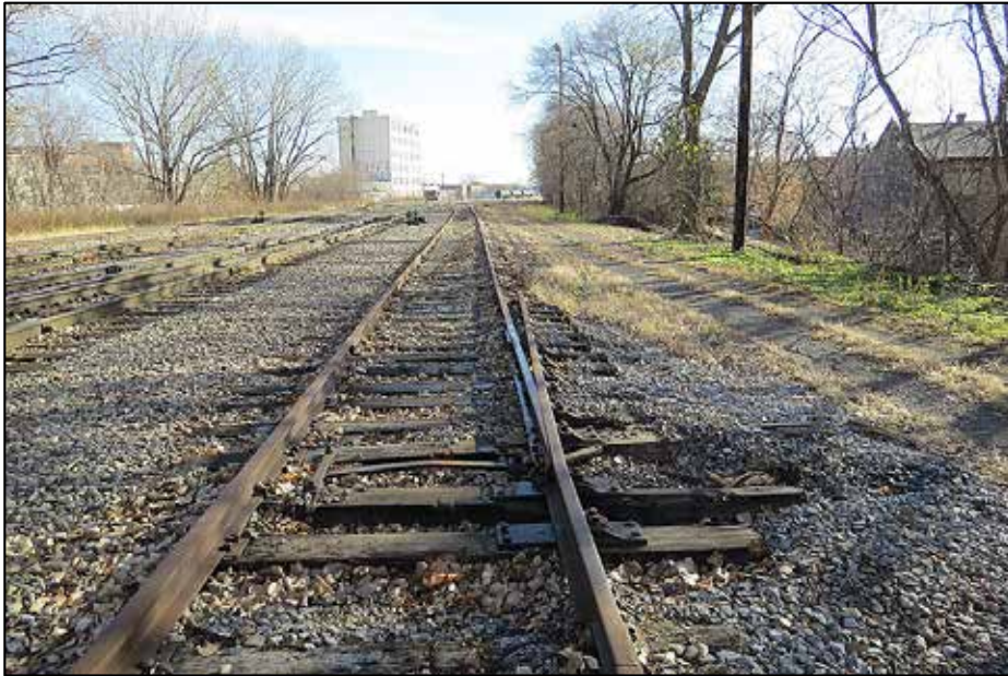
Photo 3. Switch point derail
