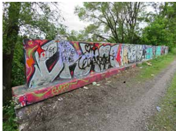
Photo 8. Graffiti on bridge railings
